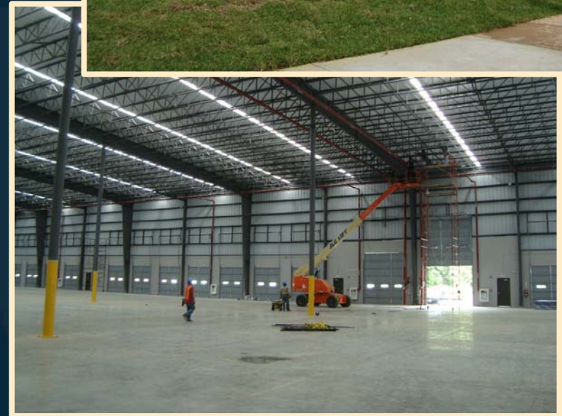
3PL Panamericana is now working on its interior finish. They plan to open in September
